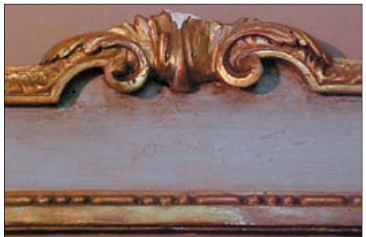
The plaster ornamentation on the mirror was chipped or missing and needed to be re-created.
